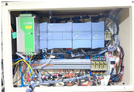
Fig. 4. PLC Cabinet Interior
